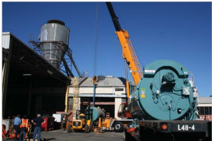
The new CBEX Elite waits on the truck bed (foreground) as the old boiler is removed
