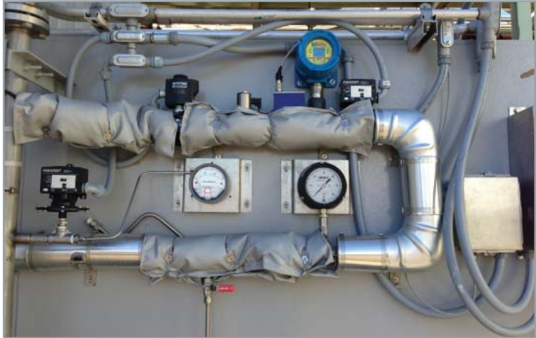
The new Anhydrous Ammonia control system for SCR
