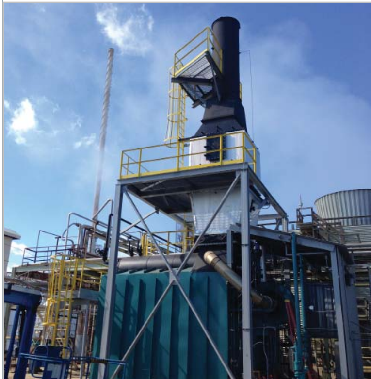
Final upgraded boiler with SCR system and new platforms, ladders, and grating
