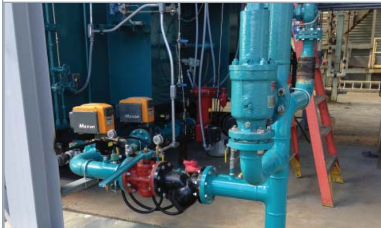
A completely new gas train was designed to meet current code and safety standards
