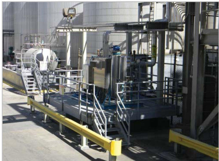
The Aqueous Ammonia skid for the installed SCR system
