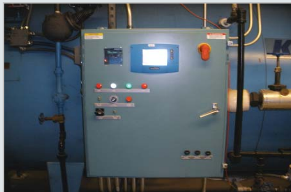
New burner control panel with Honeywell parallel positioning controls
