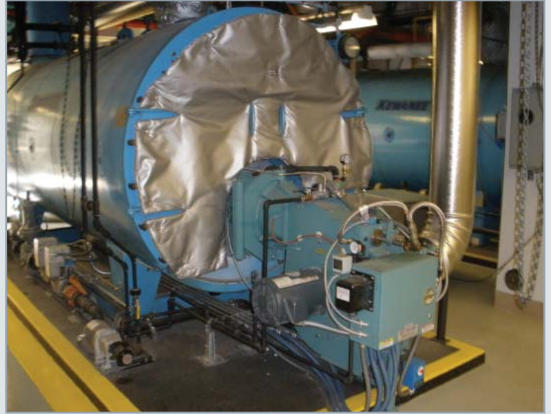
Kewanee Boiler with new burner
