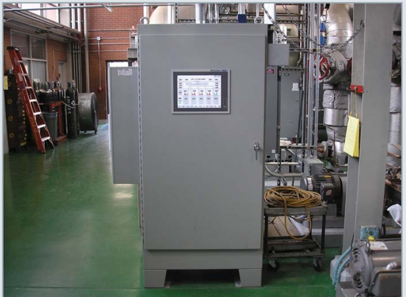
The Master Panel offers a computer touch screen for controlling equipment in several buildings
