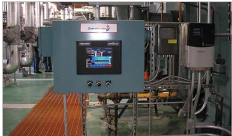
Four CB Hawk 4000 conversions are controlled manually or by the master panel through Ethernet and ModBus communications
