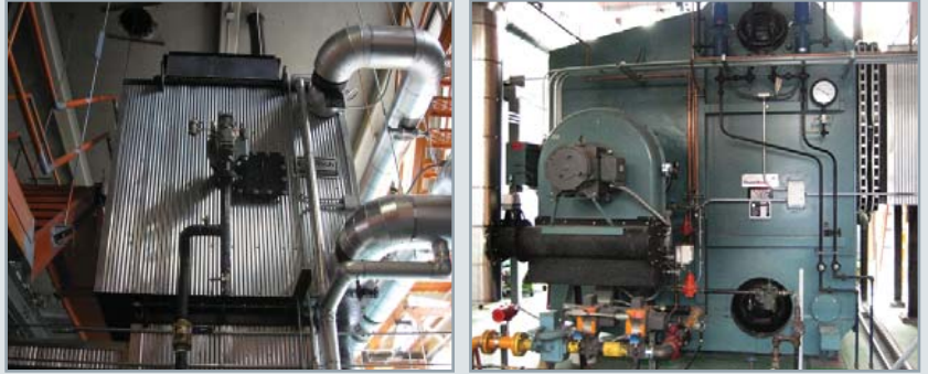
The E-Tech Economizer (left) and Nebraska Boiler (right) installed as part of this project
