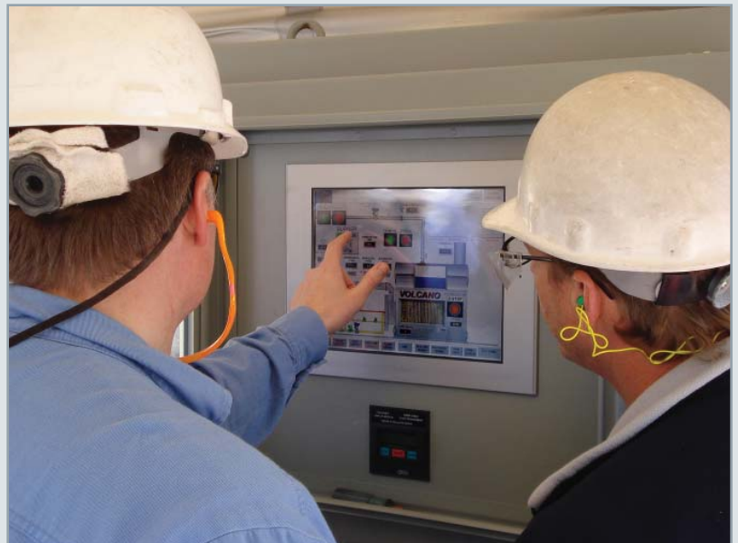
The control system panel on the final installation
