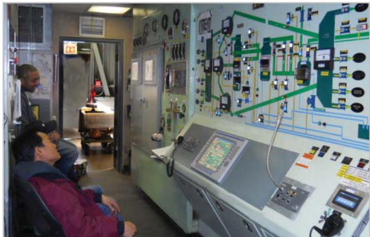
The fully completed operator control panel
