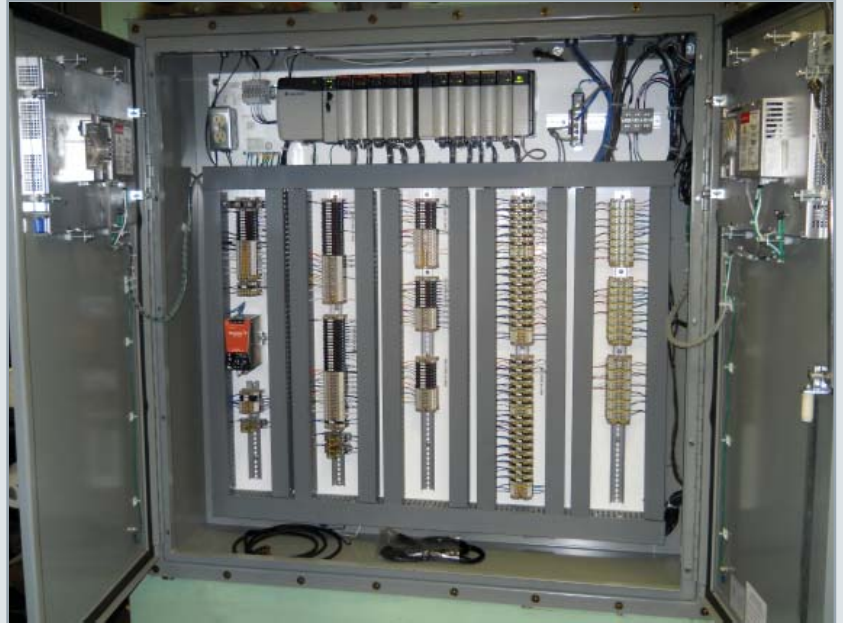
The final installation of the Controls Combustion System Panel (CCS) that controls the multiple burners of the boiler and steam generation functions
