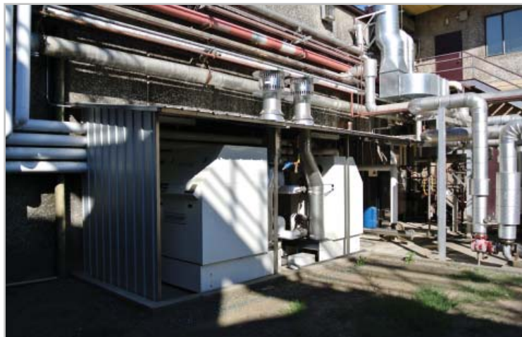
Two Cleaver-Brooks Clearfire boilers were integrated into the winery process
